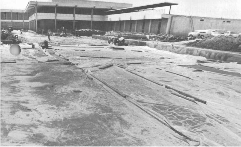
Photographed in early June, first phase of new Santa Clara Division plant still had several months to go in construction although portions were occupied and in operation by large contingent of people from former F&T. Foreground will become a large reflecting pool providing a secondary water supply for fire protection as well as an attractive setting. Eventually the roof will become a recreational patio. Exterior walls feature precast concrete panels faced with brown-hued crushed rock.
